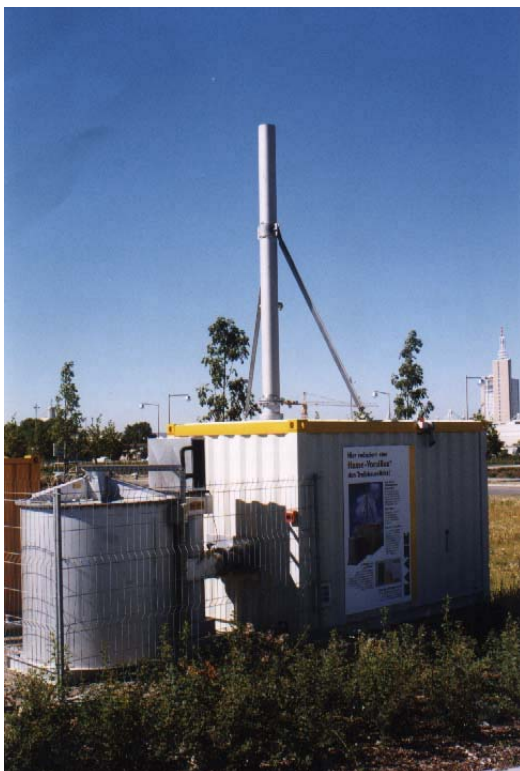
Figure 5: VocsiBox ® for the Bremerode Landfill Site, placed on the parking lot of the Hanover Exhibition Center
